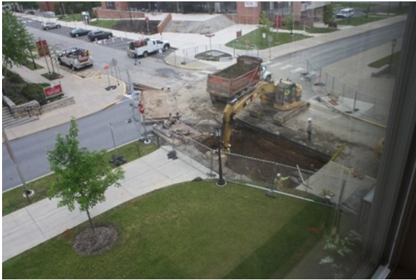
Installation of new condensate line across Pratt Drive and Maple Street intersection
