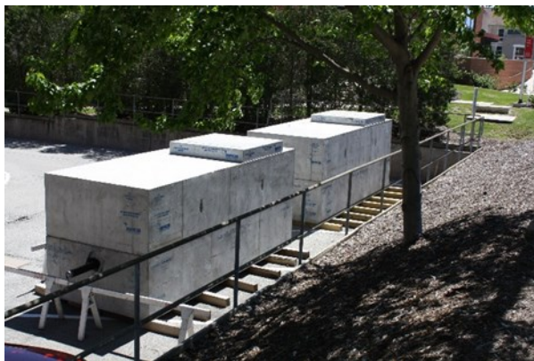
Two new water vaults staged for installation adjacent to the Cogeneration Plant
