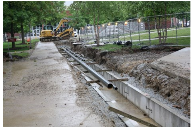
New steam and condensate lines being installed adjacent to Eberly College of Business
