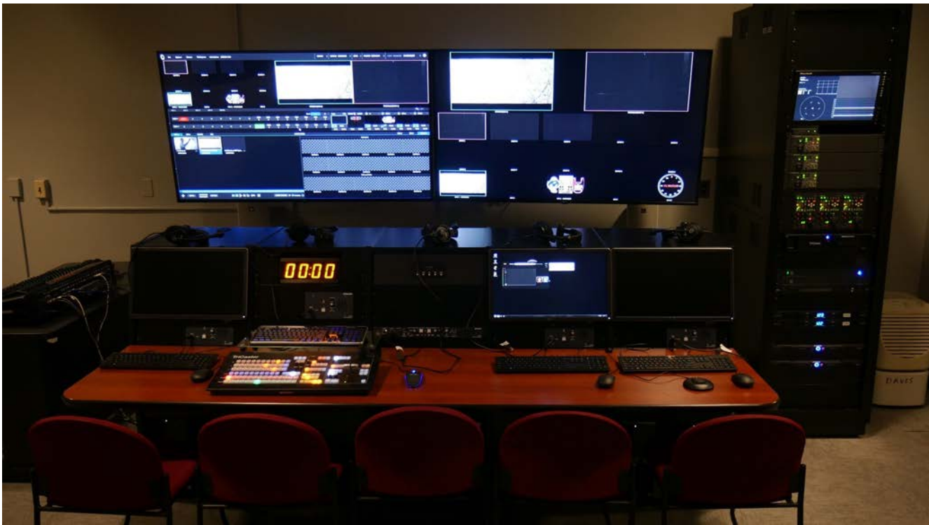
New Television Control Room
